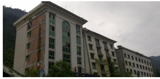
Figure13. Case 4. Leaning building. The building is Qushan School, which is next to the Beichuan Police Station.
