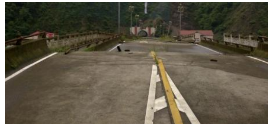
Figure15. Case 5. Xiayu Bridge, broken because of distortion from valleys.
